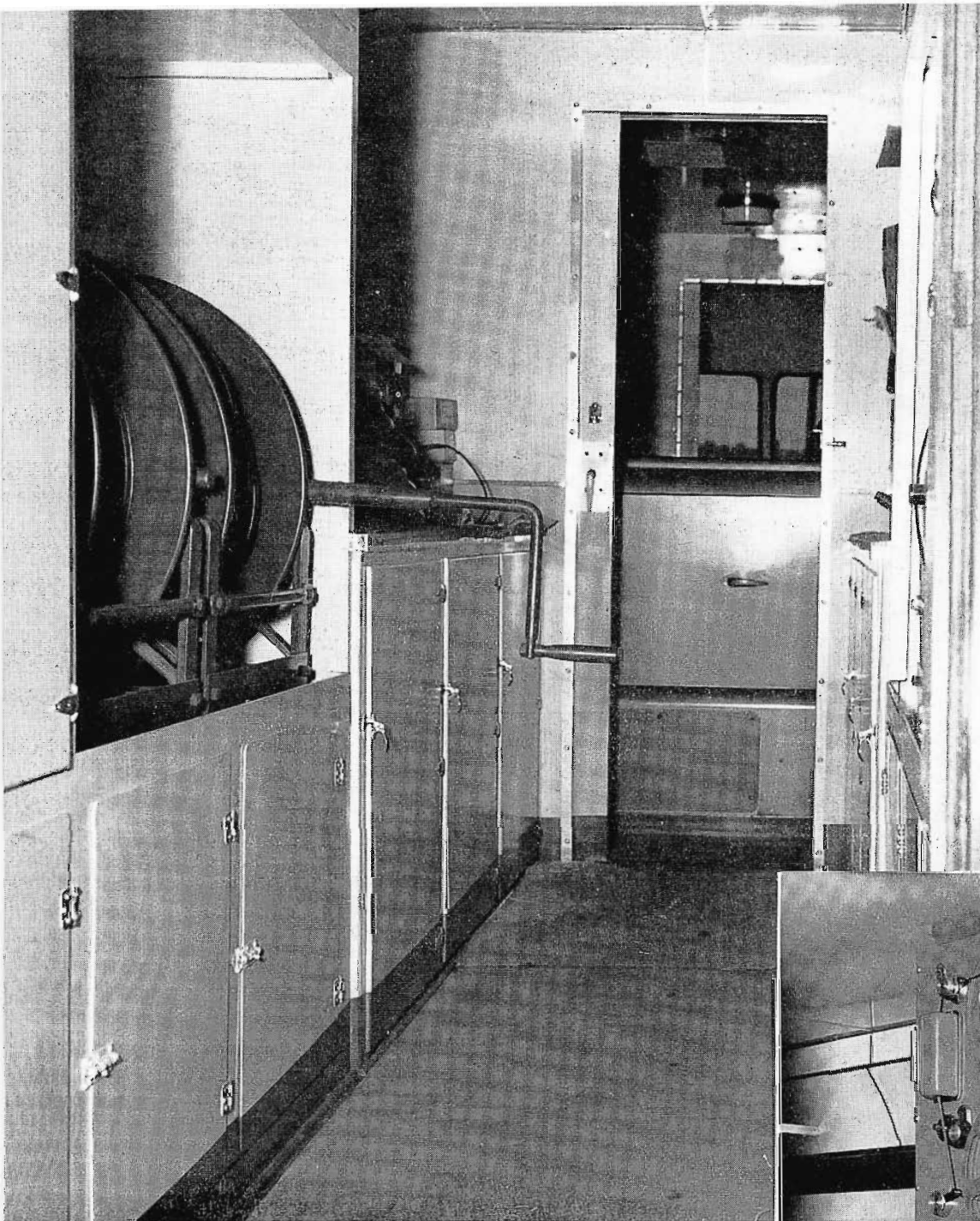
VIEW through the rear doorway of the transmitting power vehicle. Cable reels at left (and right) of corridor are for storing camera cables and power cables. Repair benches can be seen forward of the reels, and one of the gas-engine generators is visible in the next compartment behind the driver's compartment.
